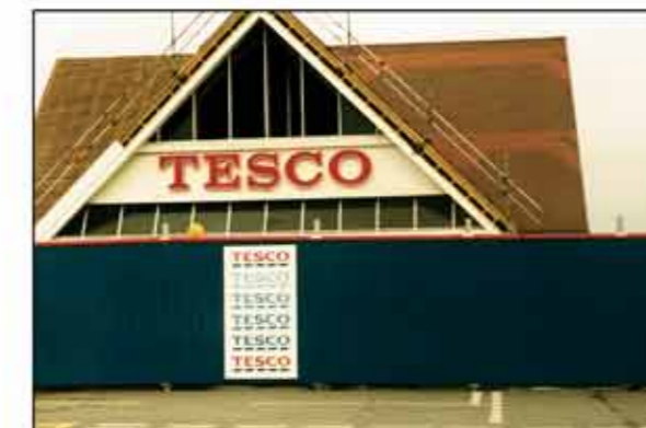
Steelhoard has been reused on a number of occasions during refurbishment and new build to conceal construction activities.
