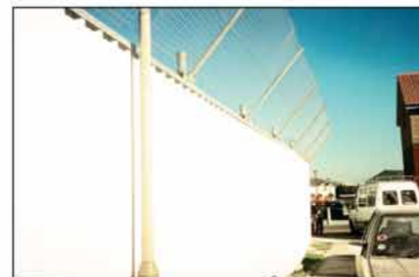
This site was customised with a welded mesh topping to meet clients' requirements.
